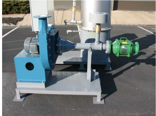
ID BLOWER WITH DILUTION FILTER AND FLAME ARRESTOR
